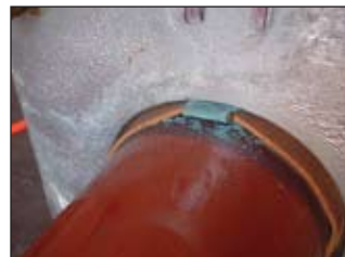
Corrosion to earth shim of CT
