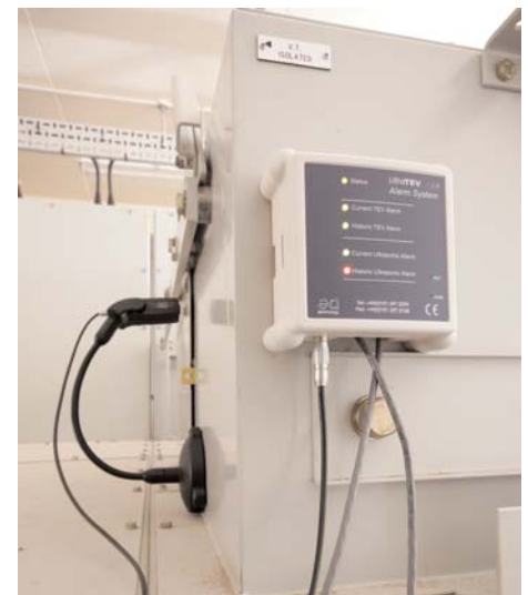
The Ultrasonic Sensor and Alarm Node
